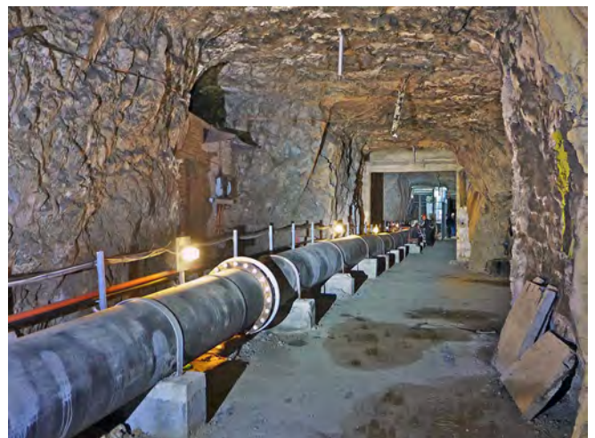
Beefsteak Magazine: a major water pipe now runs through the access tunnel
